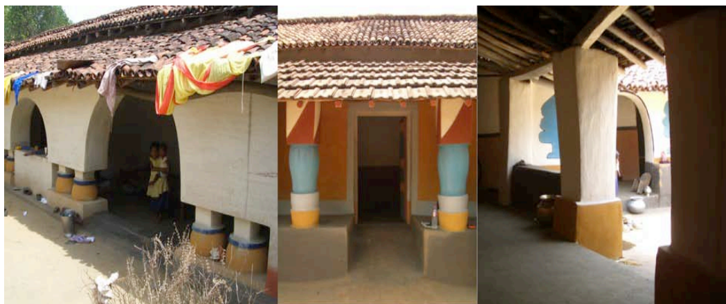
Fig. 9: Sculpted columns in different houses in Mahotabeda village (Image source: Dhaval Shah)
