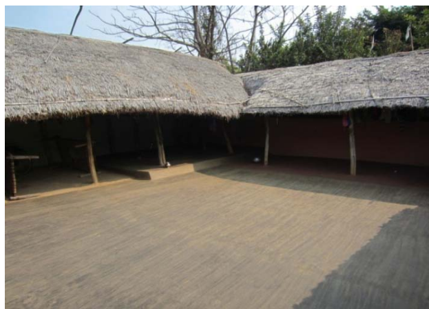
Fig. 4: Floor plastering in internal courtyard. (Note the horizontal strokes visible in plastered floor)
