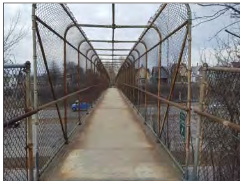
The existing Grotto St bridge will be repaired and renamed in honor of the value of social interaction. Photo Credit: Hannah Ramer
